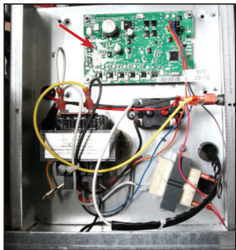
An Automatic Top Off Board, or ATO, (see arrow) monitors frypot oil levels and opens valves and runs a top-off pump to move oil from a JIB to the low frypot. The ATO board is housed behind the JIB along with transformers and a relay related to the top-off system. The McDonald's box may hold a LON board (eliminated in December 2014), a device for internal controller-based monitoring of the complete fryer system. The vats (above) are equipped with ATO sensors to monitor oil levels.
