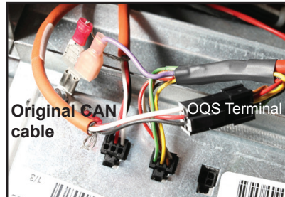
The sensor is wired in series with the CAN bus. The existing CAN cable is disconnected from the second controller from the left and the sensor plugged in. The OQS sensor cable is shown on the right: black terminal to existing CAN; gray to controller and ground.
